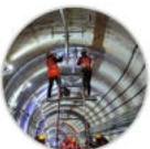
Electrical engineering grounding measurement
